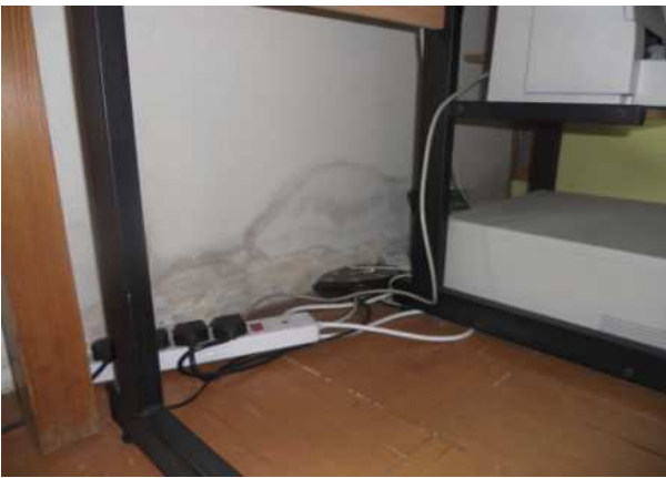
Example of rising damp
