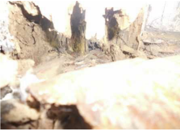
Dry rot damage on balcony post
