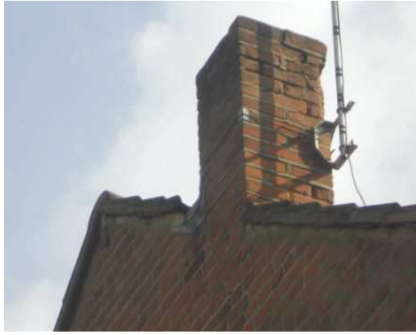
Friary Chimney damage
