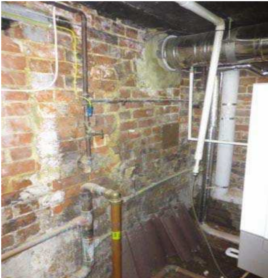
Weeping wall and damp damage in the Boiler room under the Narthex
