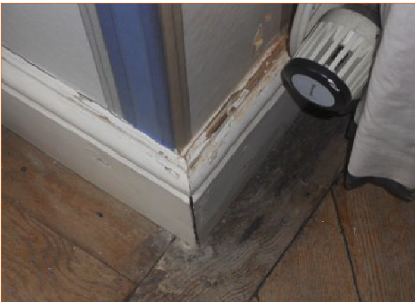
Damp patches from leaking radiator
