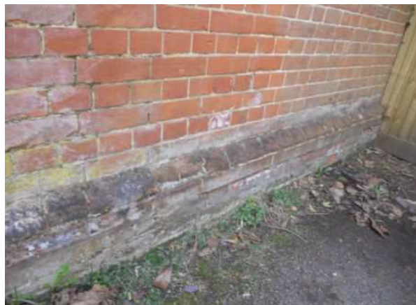
Damp Proof course damage – rising damp
