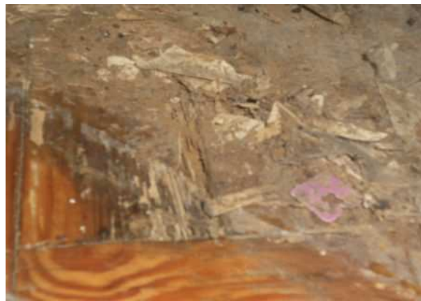
More Woodwork damage in the Friary
