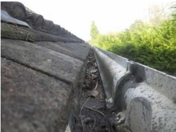
Damaged roof gutters
