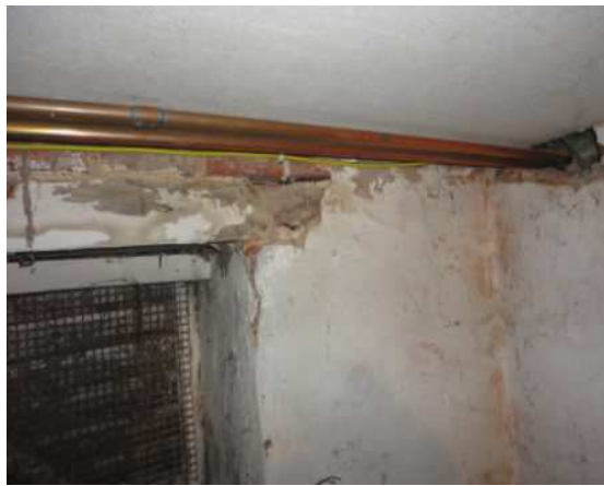
Woodworm damage on window support lintle
